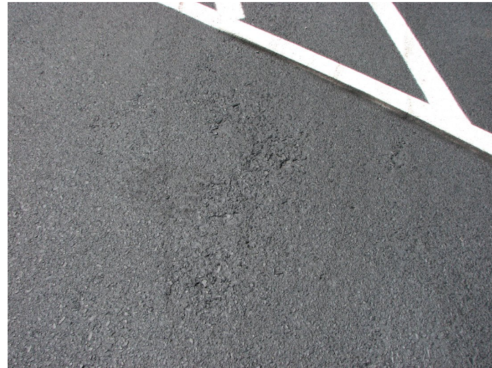
Rough areas of existing asphalt, similar to a few in the Mineral Springs lot, adequately filled
