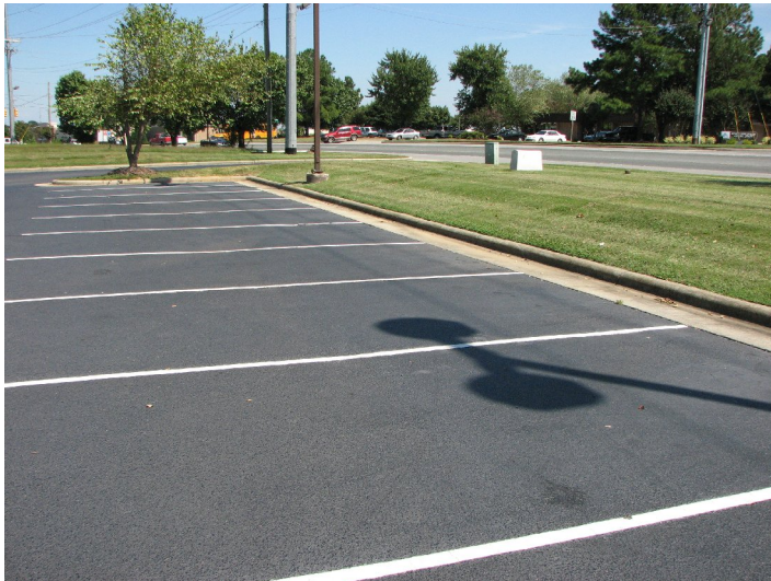
Most parking spaces are undamaged, and sealcoat application is very uniform
